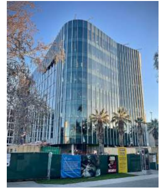
Interdisciplinary Sciences Building - under construction and part of the goal to Rebuild and Renew
